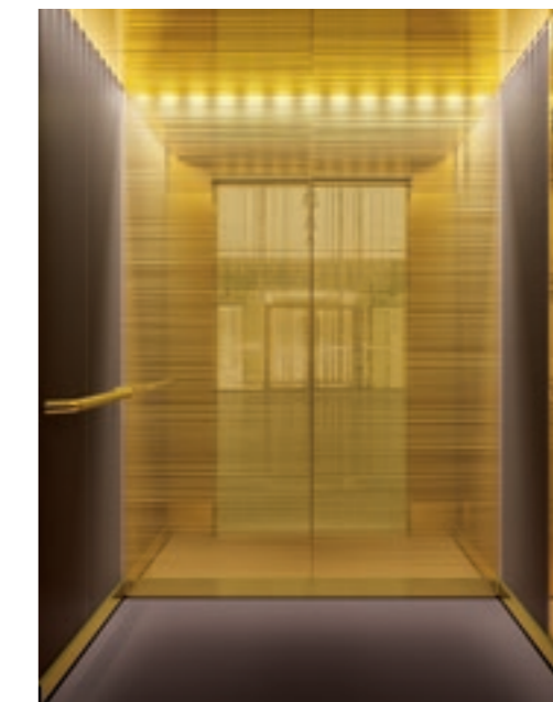
13003 Ceiling: CL181 Vegas Gold (S52) golden mirrored stainless steel, Wall B: Wenge (L221) real wood laminate, Wall C: Golden Bamboo (E54) etched steel, Wall D: Wenge (L221) real wood laminate, Floor: Brass Brown (SF33) composite stone, Car Operating Panel: KSS 670 Golden mirror (HTIN) polished stainless steel faceplate, Handrail: HR66 Shangri-La Gold (S51) golden brushed stainless steel, Skirting: Shangri-La Gold (S51) golden brushed stainless steel
